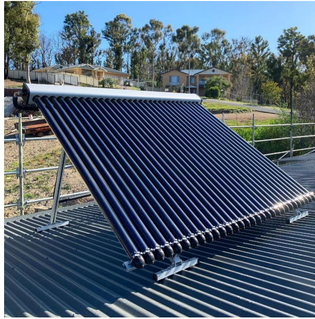
Evacuated solar tubes
